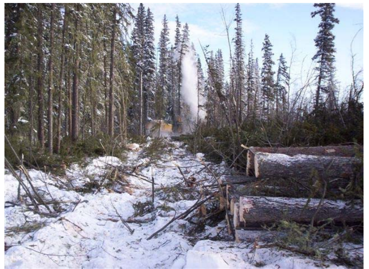
Photo #1: Feller buncher working along the face of the block opening. Note that the snow acts as a cushion for the machine and leaves no site disturbance.
